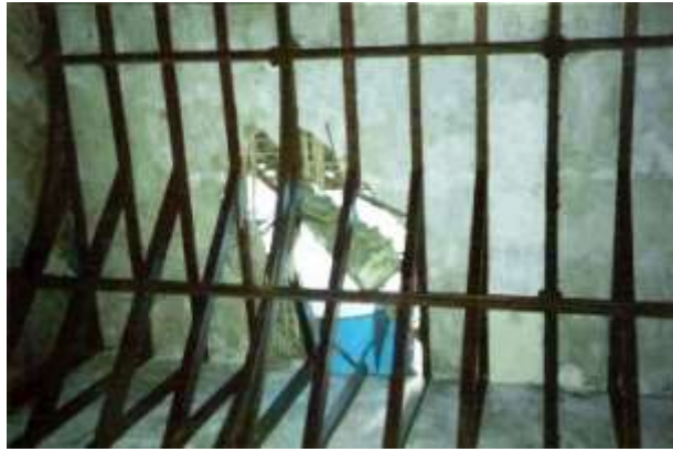
The pinnacle precariously perched! December 1990
